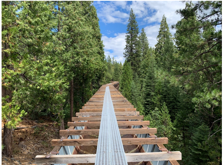
Trees encroach on the South Yuba Canal, NID's primary water conveyance infrastructure. The project will focus on removing trees to protect against wildfire.
