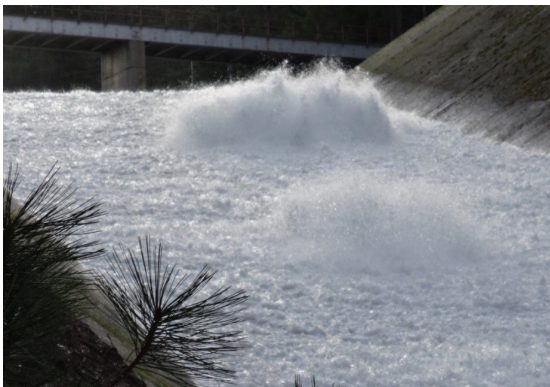
Damage caused by spalled concrete
