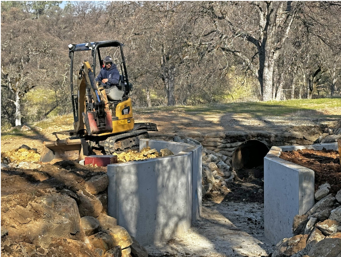
An NID Utility Worker puts the finishing touches on the construction of a check structure in Newtown Canal.
