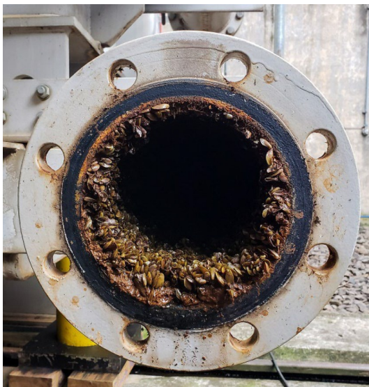
Golden mussels colonize a water pipe at a hydroelectric plant in Brazil in 2021.
