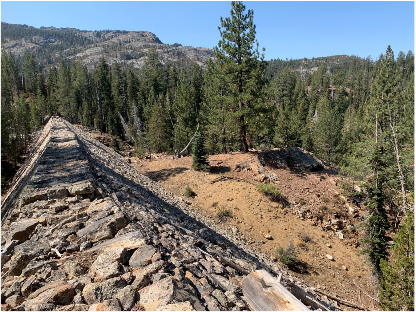
Figure 9. Remains of East Dam looking southwest (Source: Nevada Irrigation District, Cameron Townsend).
