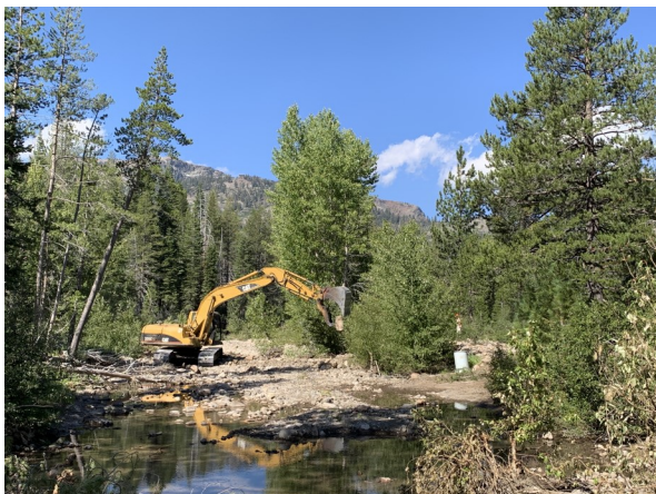
An excavator constructs in-stream debris jam structures in the Middle Yuba River
