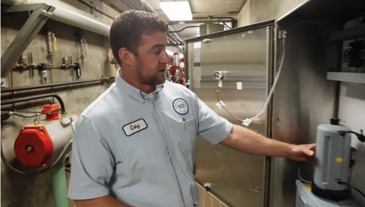
The NID Water Treatment Supervisor uses a turbidimeter to measure water clarity and ensure safe drinking water.
