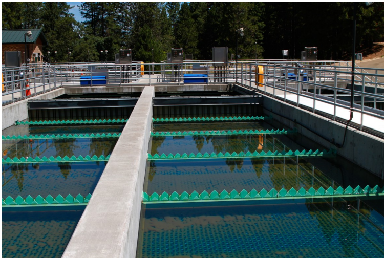
Settling and filtration basins at the Elizabeth George Water Treatment Plant help ensure safe drinking water.
