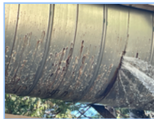
South Yuba Canal Leak.JPG
