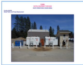
Diesel Tanks and Pump
