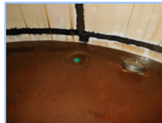
Rusted wall inside tank
