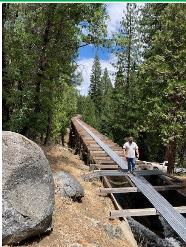
The NID Environmental Resources Technician examines the landscape along the South Yuba Canal, where trees encroach on the structure from both sides.
