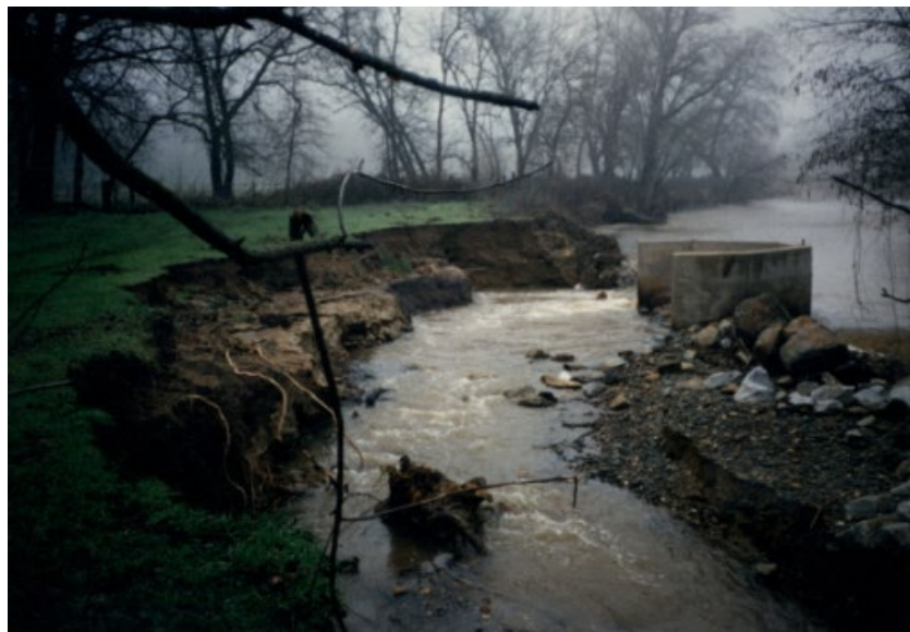
Figure 1-2. Extensive erosion on the north bank caused by high flows in 1997. Photo provided by NID.
