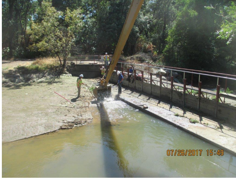
Figure 1-4. Placing riprap in scour hole upstream of dam following winter 2017 floods. Photo provided by NID
