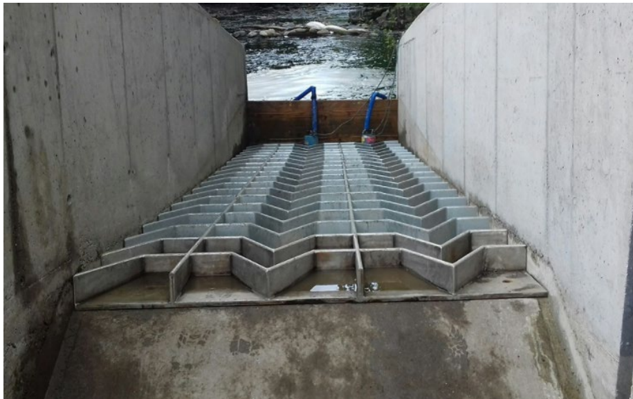
Figure 3-6. Larinier fishway looking downstream. Note the vertical, smooth side walls, and the wide, baffled base. Photo credit: Aquatic Control Engineering
