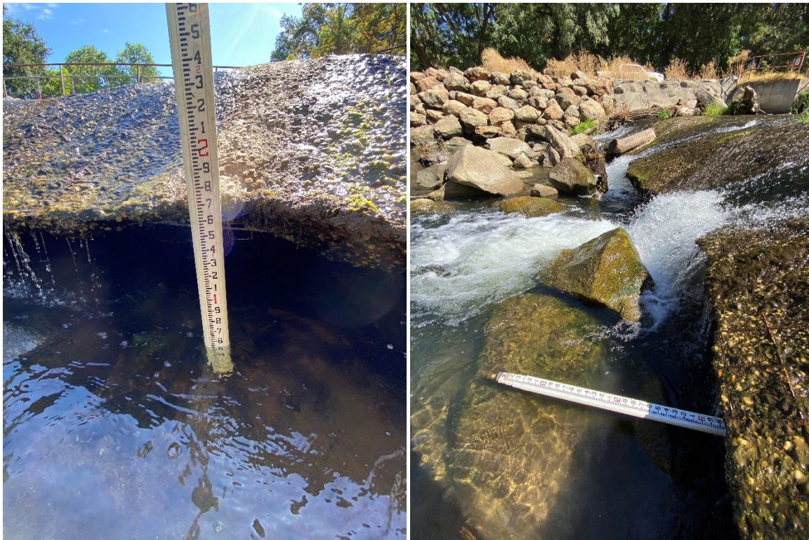
Figure 2-1. Erosion under the dam apron as of September 22, 2020. The apron was constructed after the 1997 flood, as shown in Figure 1-3. The photo on the left shows the apron perched approximately 1.5 feet above the downstream channel bed. The photo on the right shows that the scour hole extends approximately 11 feet under the dam; the wire mesh, that was originally encased in the shotcrete is becoming exposed on the apron’s surface.
