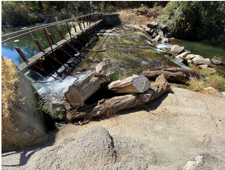
Figure 2-3. Large woody debris accumulated on the banks and the dam's apron
