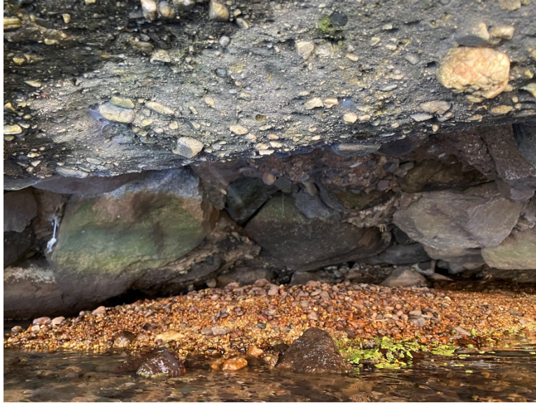
Figure 2-2. Looking under the dam apron – the foundation has eroded under the concrete encased boulders.
