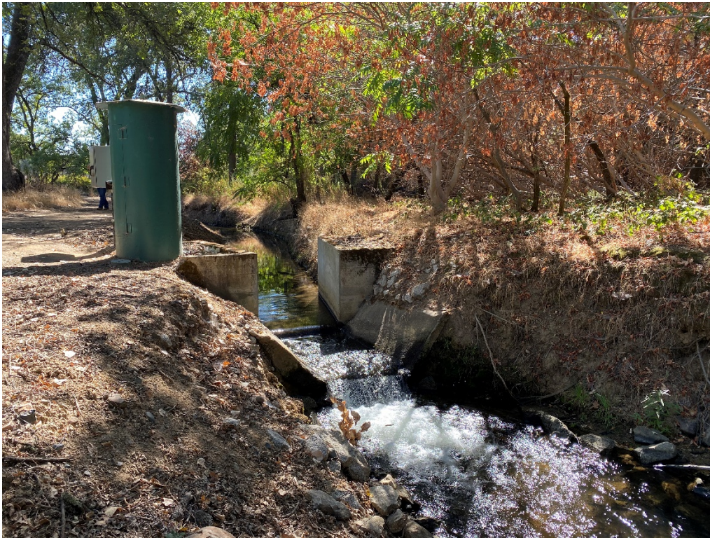
Figure 2-4. Gaging station and Parshall flume within the Hemphill Diversion. Photo source: NHC
