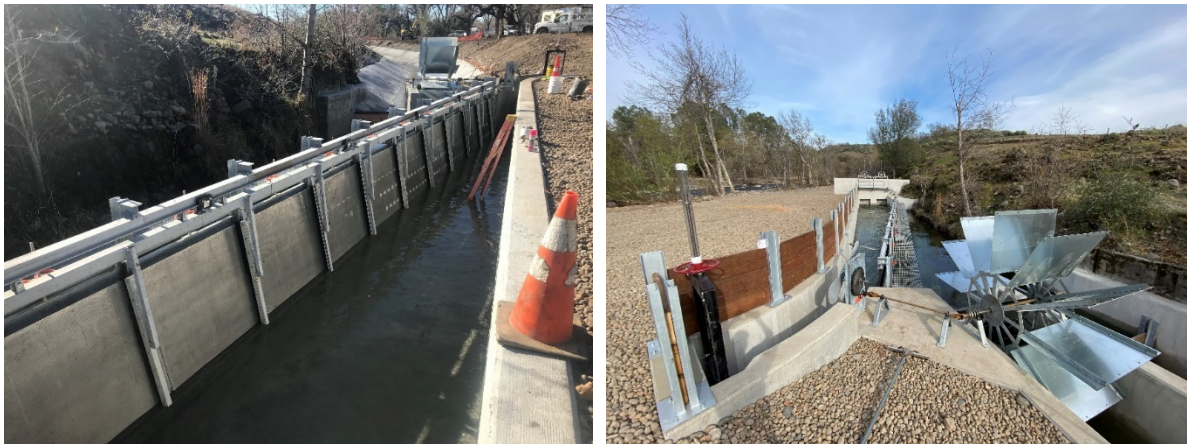
Figure 3-9. Example of a flat plate screen. NHC designed and installed this screen for Deer Creek Irrigation District in Tehama County, CA in 2019.
