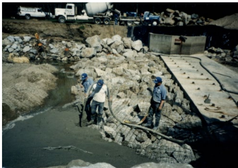
Figure 1-3. Fortifying the banks and dam apron with grouted riprap following the 1997 flood. Photo provided by NID.
