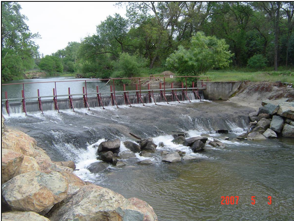
Figure 2. Hemphill Dam at beginning of irrigation season, with 3-foot tall flashboards installed.
