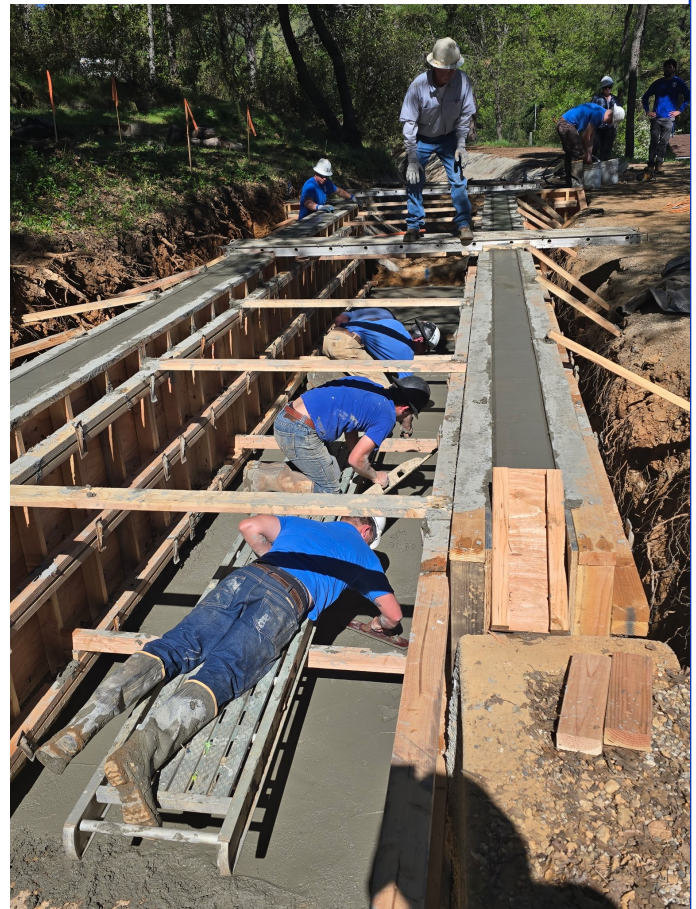
Above right: Concrete is poured into the form to create a wall for the new automated gage.
