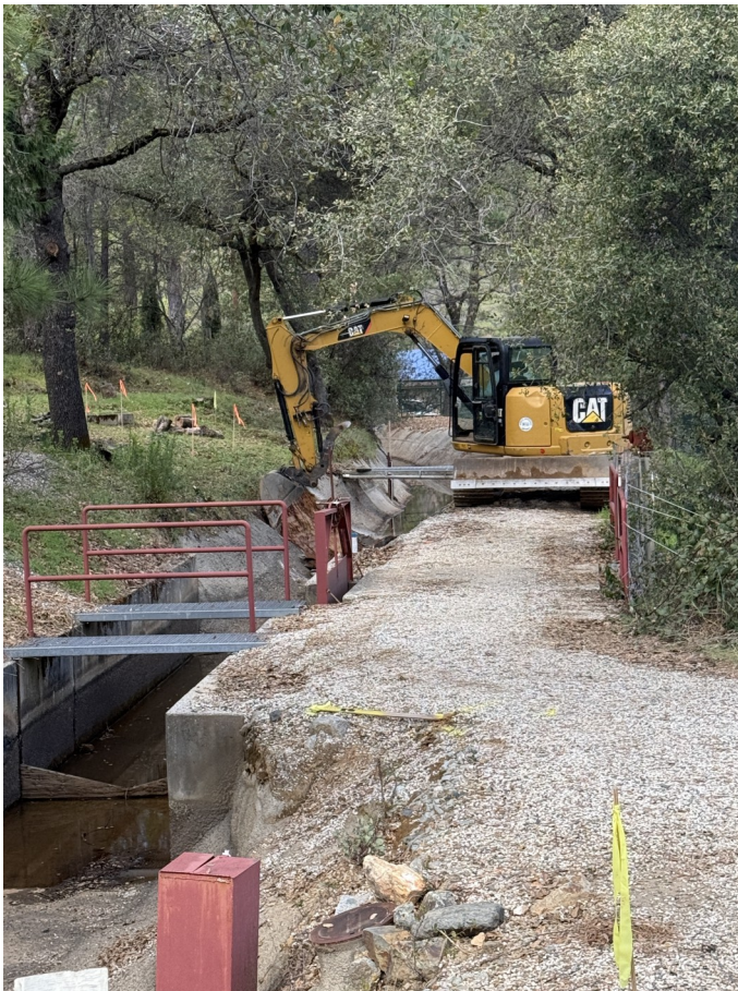
Above left: The canal is prepped for placement of the wooden concrete form.
