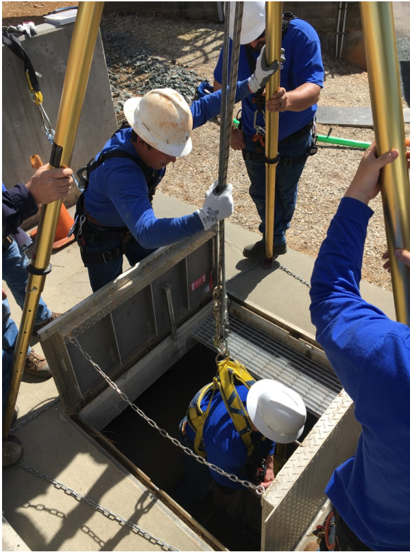
(Left) Logan Vanderhoof assists in hoisting Declan Maloney from the vault at E. George Treatment Plant.
