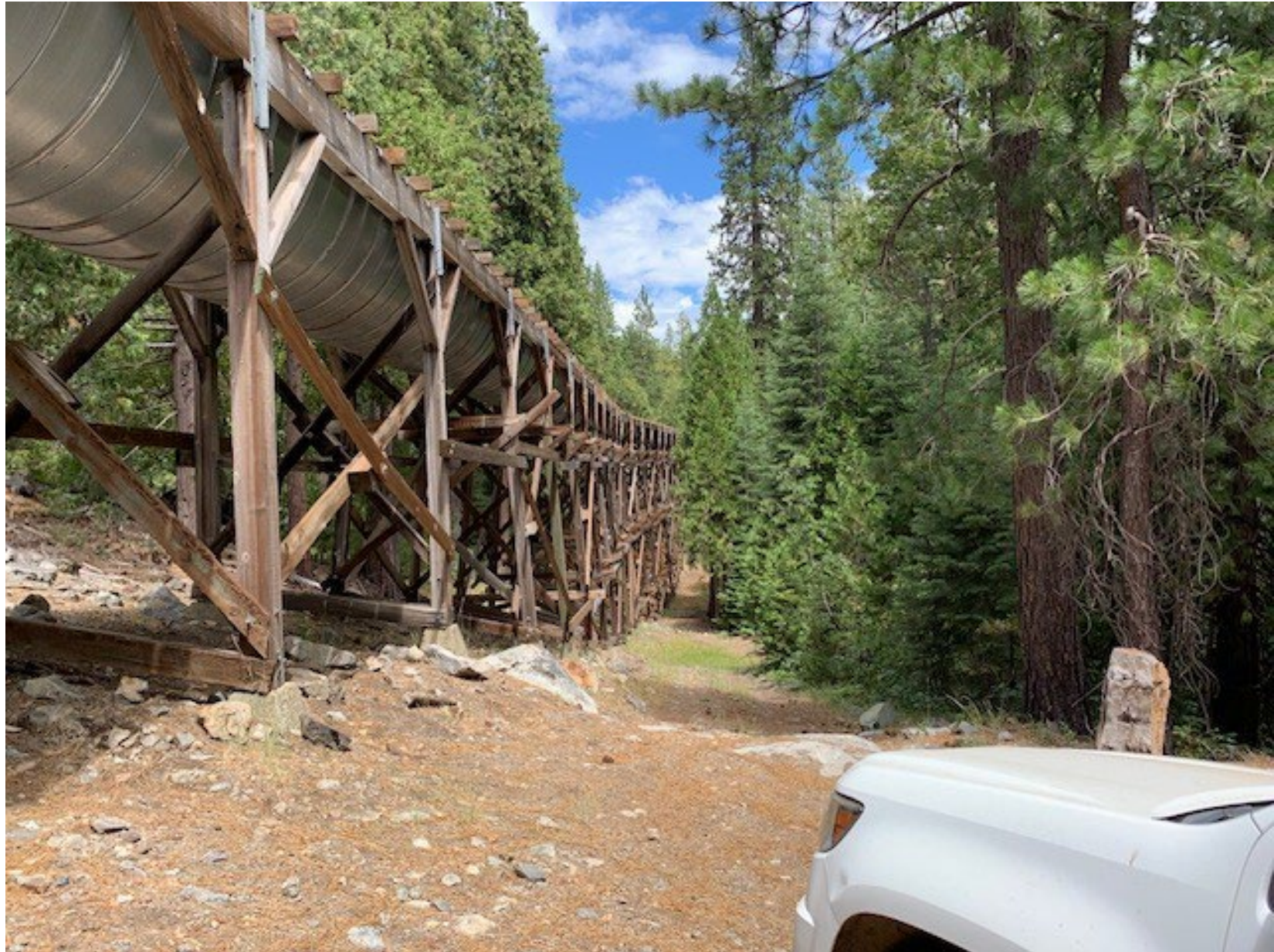
South Yuba Canal wooden supports exposed to potential wildfire
