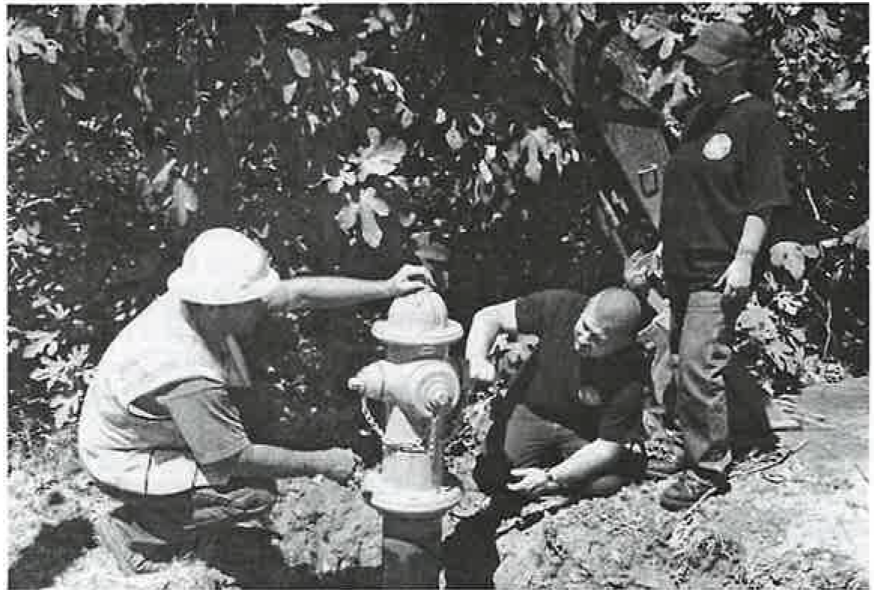
NID's Cameron Price shows a new dry barrel fire hydrant to Chris Turner and Cari Edgerton, volunteer firefighters with the Smartsville Fire District.
