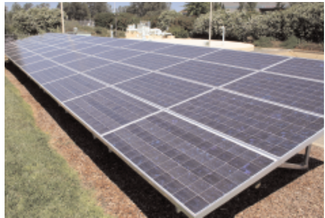
The solar array at NID's North Auburn Water Treatment Plant
