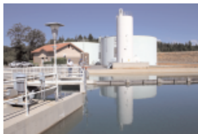
Loma Rica Water Treatment Plant near Grass Valley
