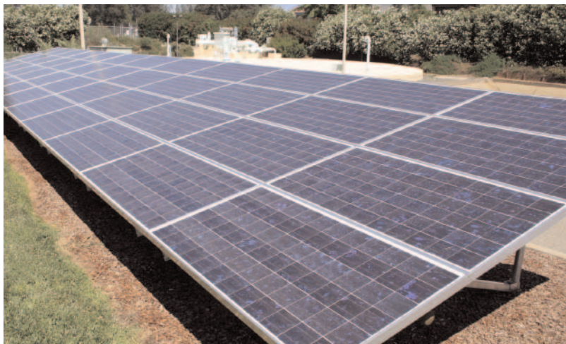
This is one of three solar panel arrays now generating electricity at NID's North Auburn Water Treatment Plant
