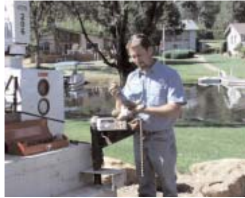
Chris Berg prepares a meter for installation at Lake of the Pines
