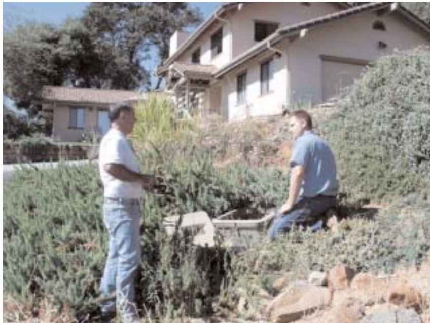
Service Crew members John Ottonello and Eric Fassler check a meter box at a Lake of the Pines residence.
